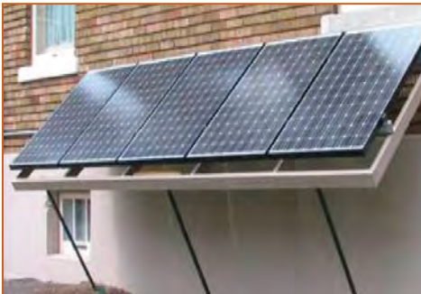
1 kW wall-mounted solar array
