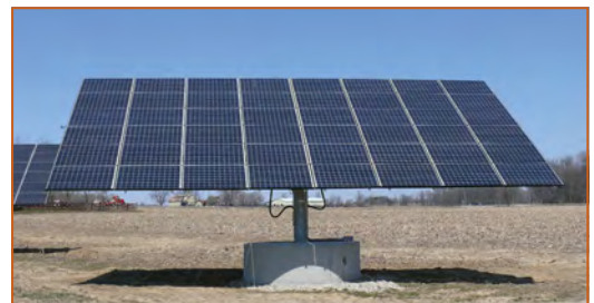
2 kW ground-mounted solar array
