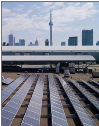
Large ground-mounted solar PV facility
